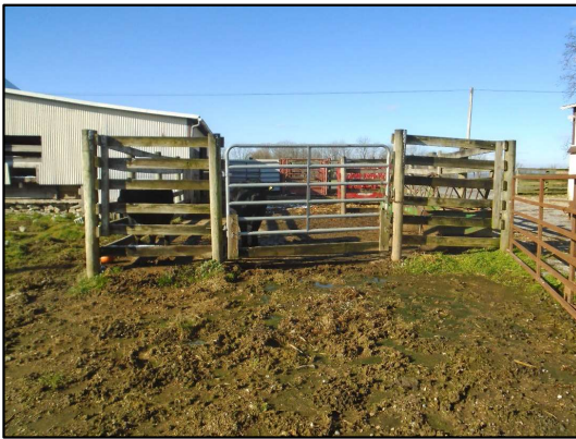
BEFORE: Severe critical runoff area with high potential for nutrient, sediment, and pathogen runoff to downslope stream.
