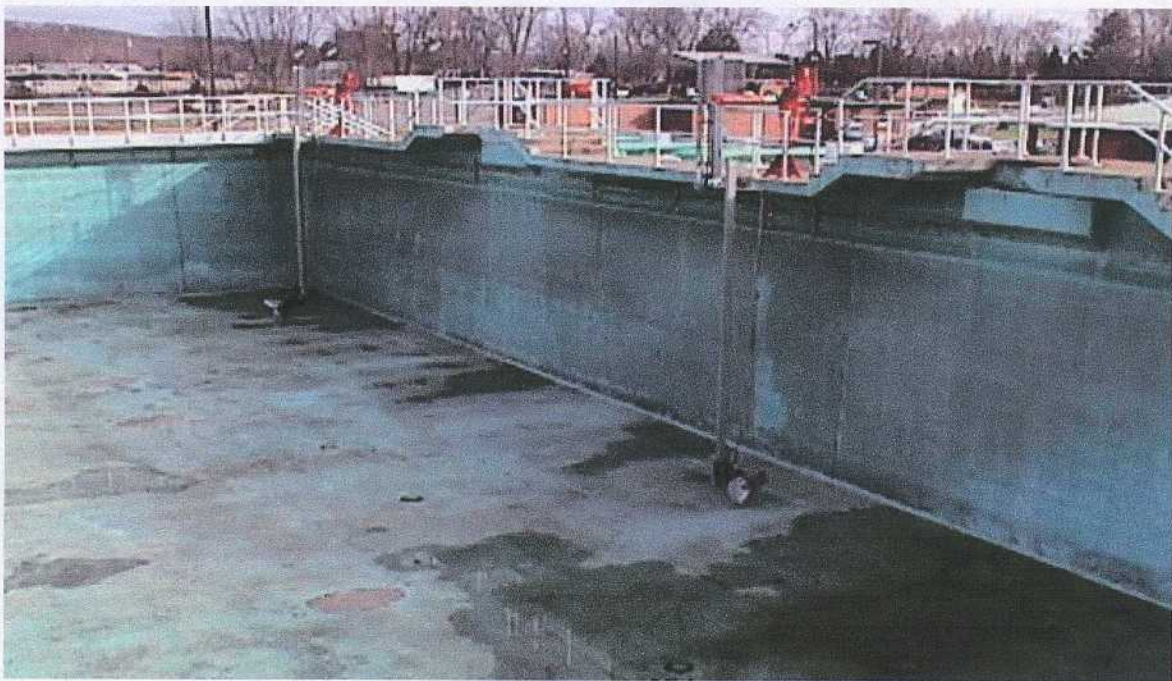
Original aeration basin converted to a BNR unit.
