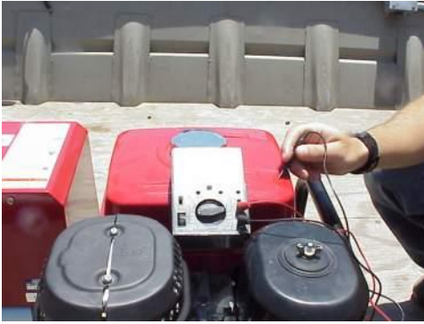
Pic. 5 – checking continuity between generator And boat hull. (NO continuity due to paint)
