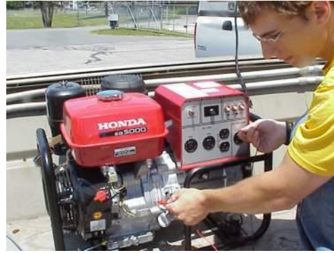
Pic. 6 – continuity check between ground receptacle contact and generator. (there is continuity)
