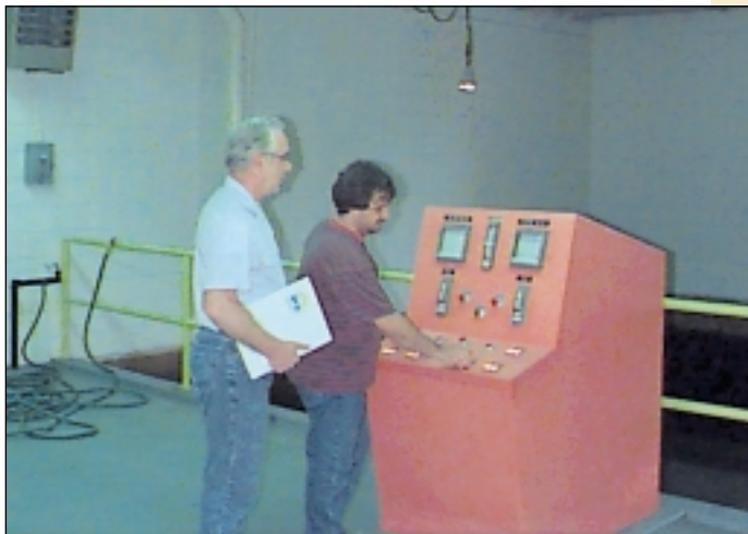
Don Greenfield (left) watches Tim Biseli, an operator at the Altoona Horseshoe Curve plant, initiate a filter backwash from the control panel.
