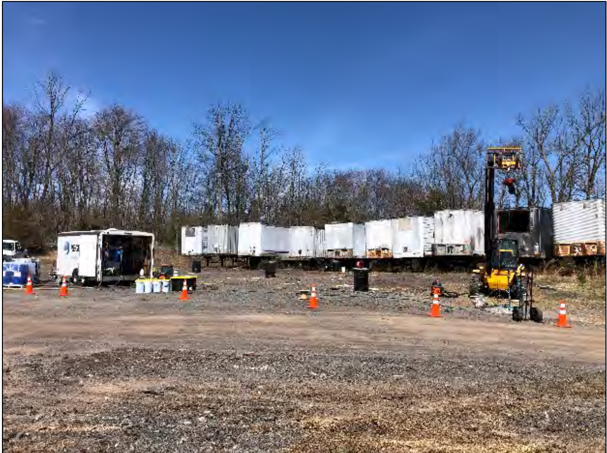
Photo 2: Injection area with RRS injection trailer Looking N
