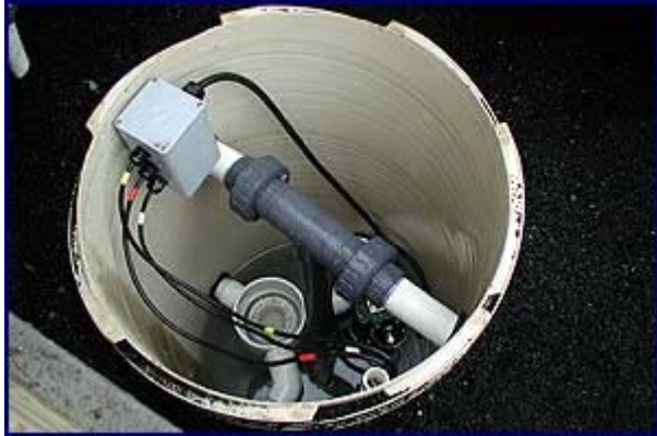
Inside the pump vault.
