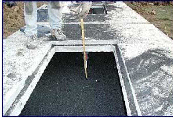
Measuring the freeboard space in one of the CO-OP RFS III's filter tanks.
