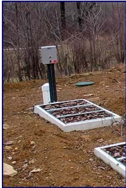
The white pipe next to the control box is the inspection port for the UV unit.
