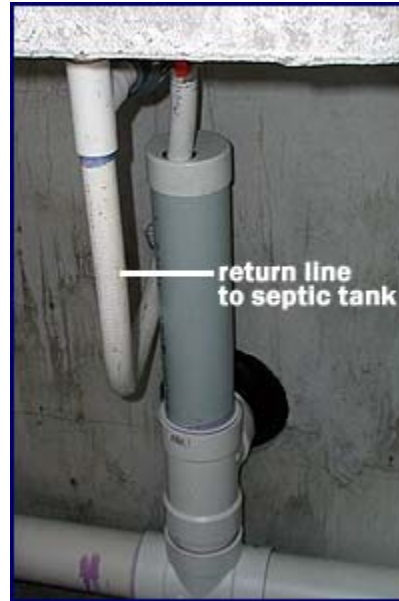
This view from inside the CO-OP RFS III tank shows where the return line to the septic tank is installed, just a few inches above the connection from the second compartment or septic tank to the CO-OP RFS III.
