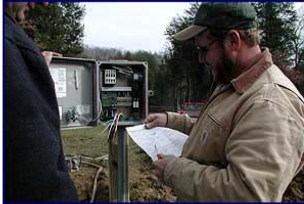
At the control box.
