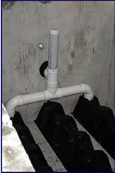
This shows the yoke coming from the septic tank into the first filter tank.
