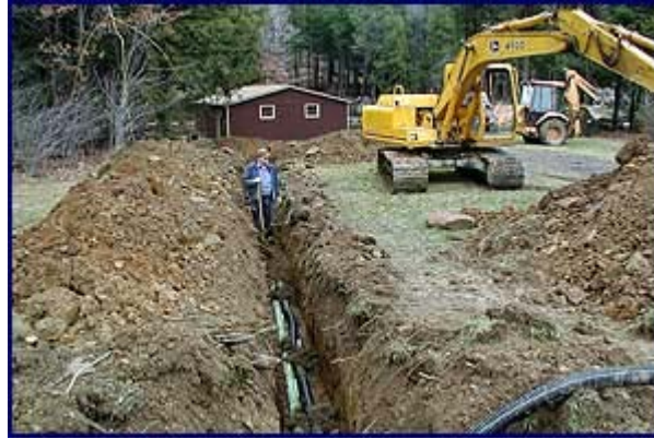
Here, septic lines installed from the CO-OP RFS III to the absorption area are ready to be backfilled.
