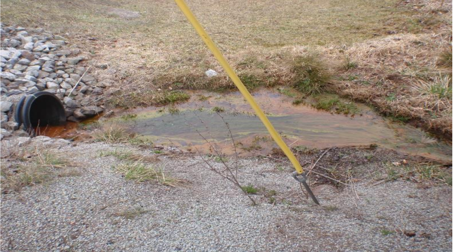
Figure 3: Cross Road Stormwater Pipe discharging to Undocumented Tributary to Oven Run.
