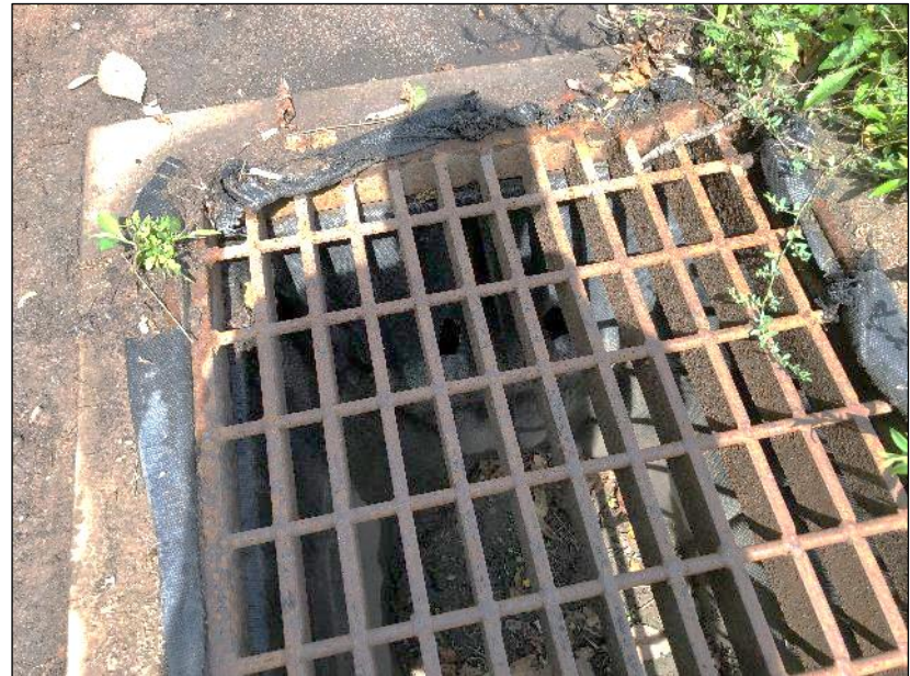
Catch basin to Outfall 009 with holes in the filter insert
