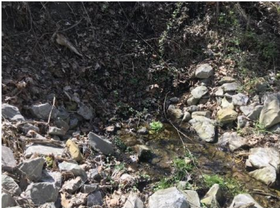
Figure 9. From the channel, downslope of the trail crossing, looking at the trail crossing (note the lack of culvert).
