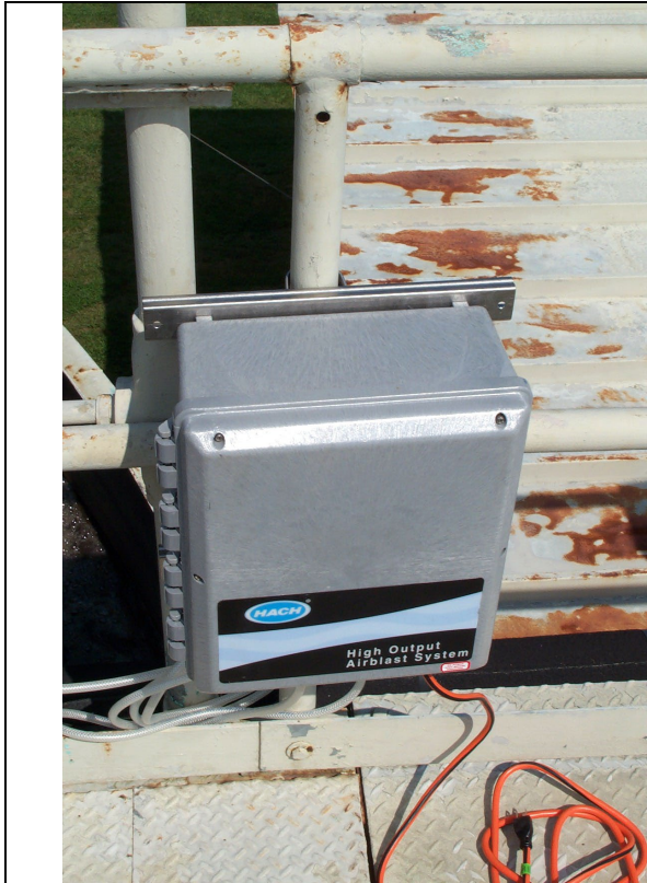
Figure F-3: NH3-N Cleaning Compressor
