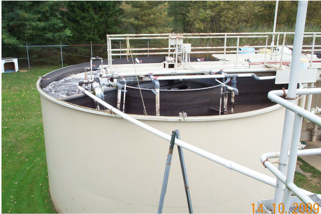
Figure M-1: Raw Wastewater Shunt to Stabilization Tank 1.
