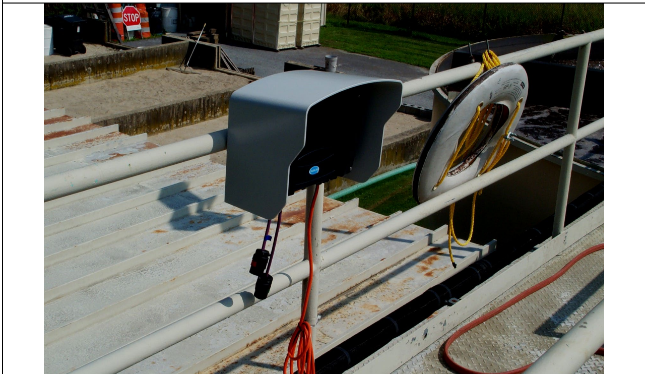
Figure F-2: SC-1000 SCADA Unit with Sunshield on Railing near Contact Tank 1
