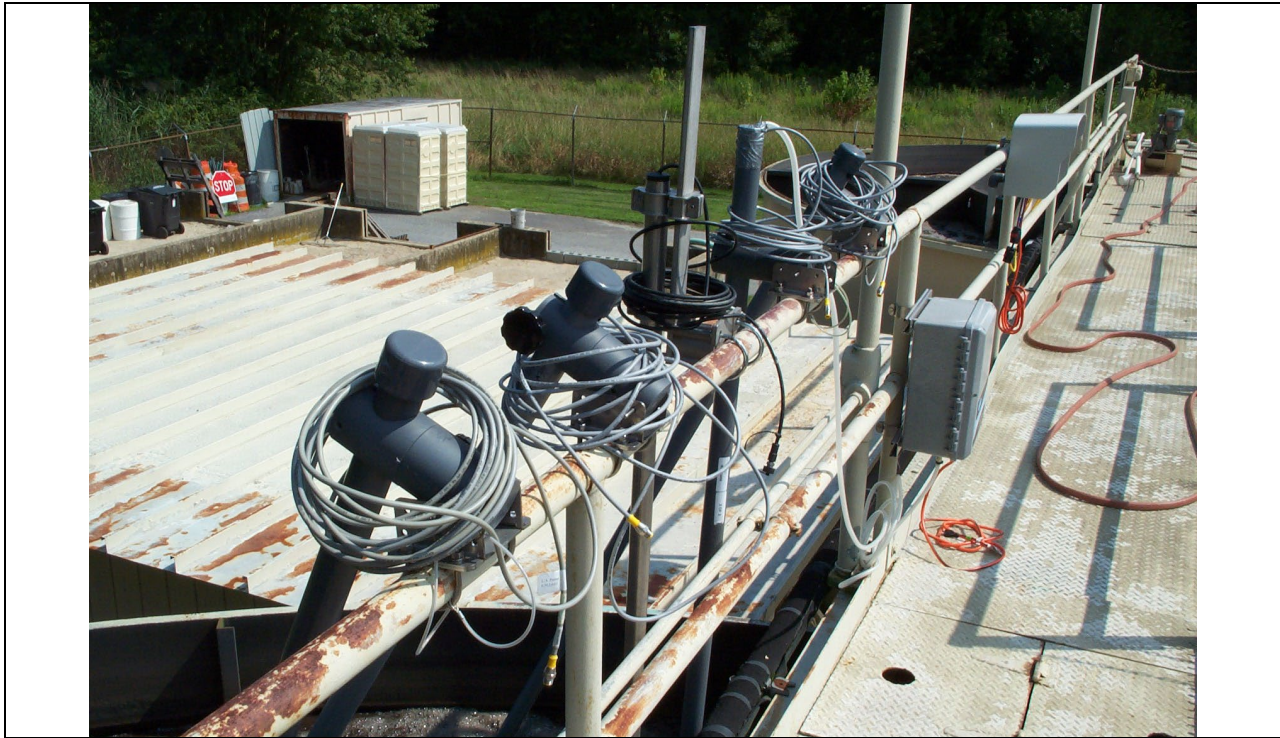
Figure F-1: Nitrate, Ammonium, TSS, DO, and pH probes installed in Contact Tank 1
