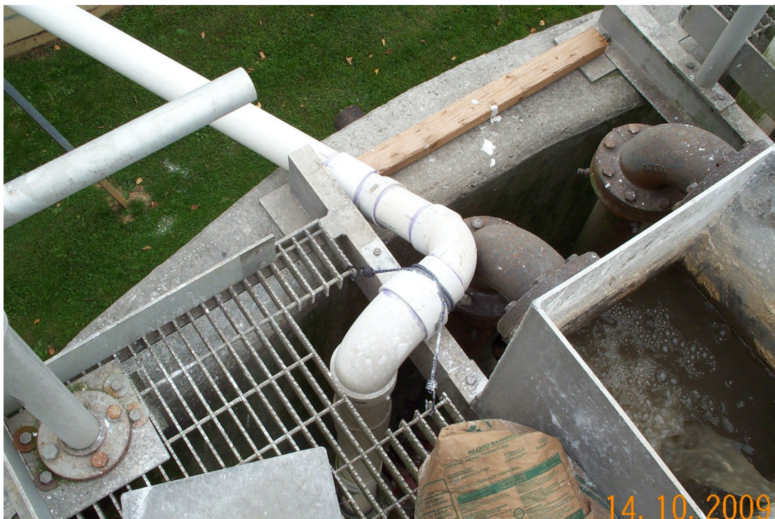
Figure F-11: Raw Shunt Connection at EQT Lift Pump Relief Line
