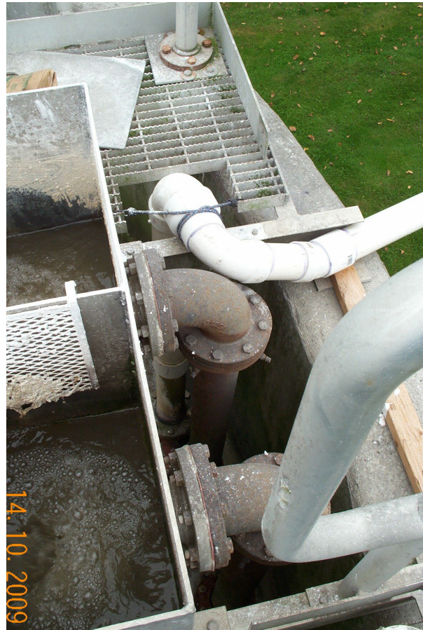
Figure 35: Another View of Raw Wastewater Shunt
