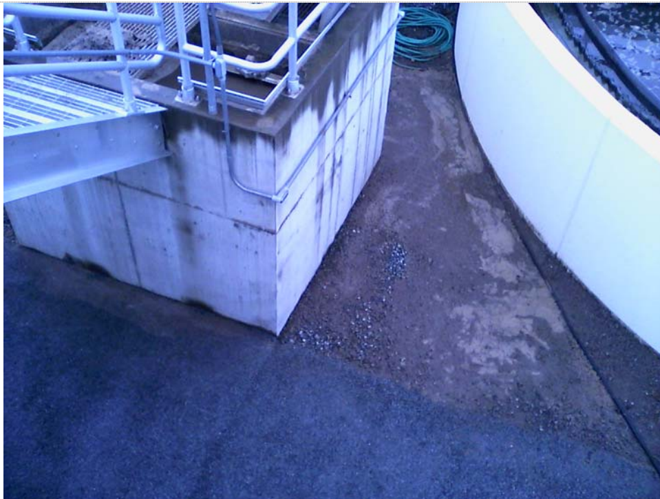
Figure 6: Evidence of line obstruction at clarifier feed splitter box.
