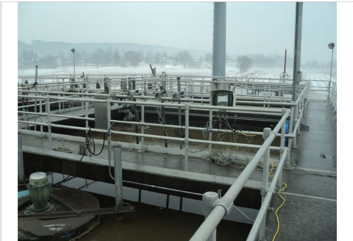
Figure 4: Probe Installation at SAR: pH, TSS, DO, and ORP; Anoxic Tank: ORP
