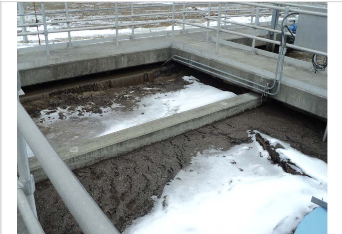
Figure 2: Scum Layer (filamentous organism reservoir) on Pre-Anoxic Tank & Phase Separator
