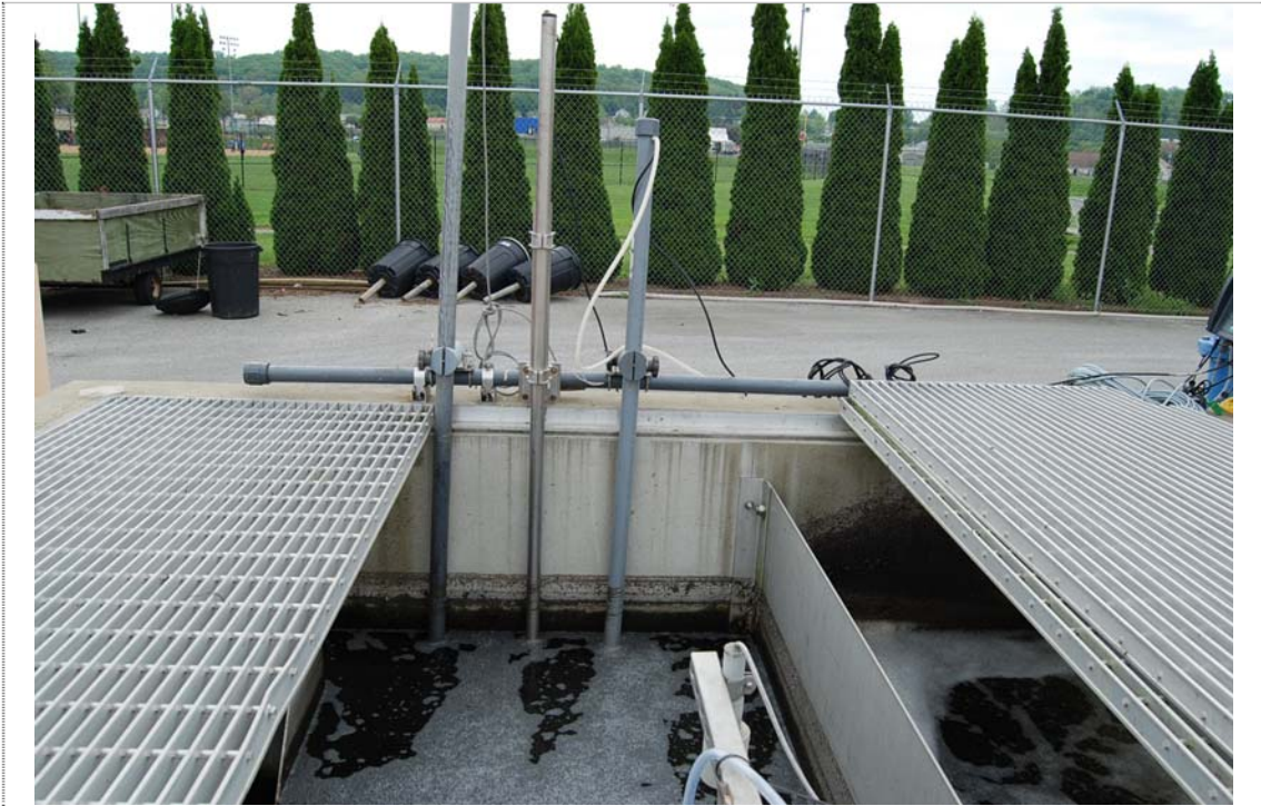
Figure 3: Probe Installation at Effluent Reaeration Tank: Nitrate, Ammonium, & DO Probes
