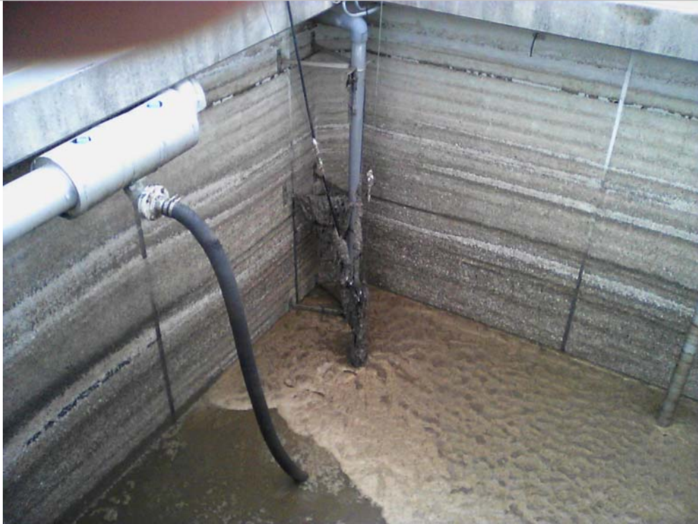
Figure 7: Example of rags accumulating in aerobic digester
