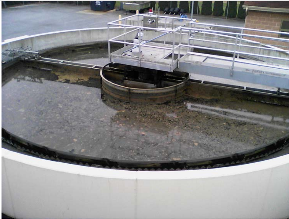
Figure 5: Secondary Clarifier inflow line was clogged by rags and taken out of service.
