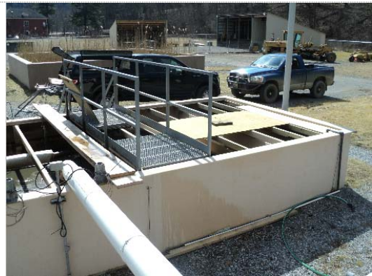
Photo 4: Influent Transfer Pipe to Anoxic Tank B
