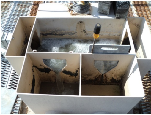
Photo 3: Influent Splitter Box with Overflow
