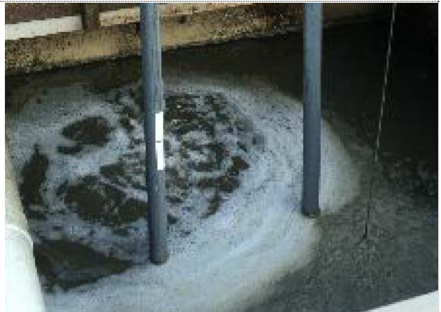
Photo 6: Subsurface air turbulence in Anoxic Tank, Train B
