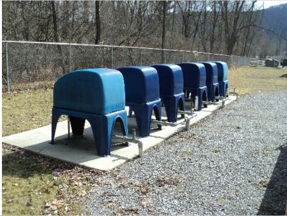
Photo 9: PD Blowers, individually piped
