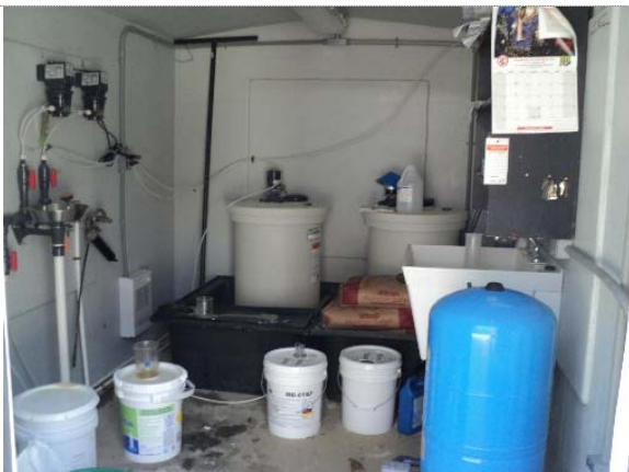
Photo 11: Unused Phosphorus Control System
