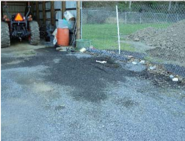
Photo 19: Oil-stained gravel by equipment sheds
