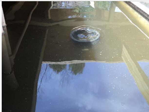
Photo 15: Unadjusted scupper / flooded clarifier
