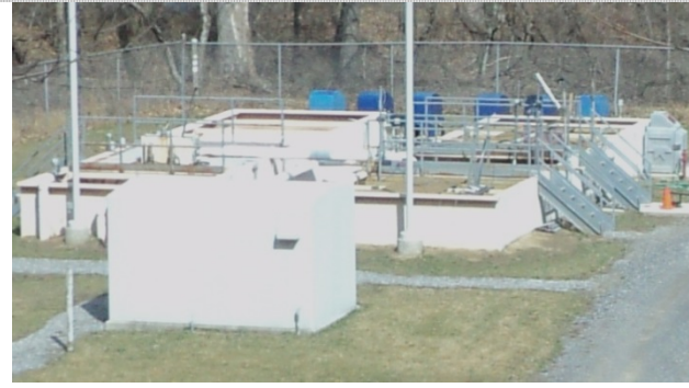
Photo 1: Purestream EA Tanks—Trains A (left) & B (right)
