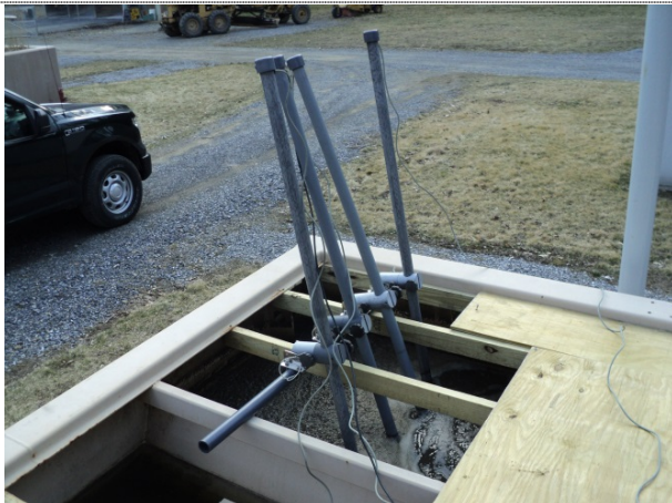
Photo 5: Probes staged in Oxidic Zone B-1
