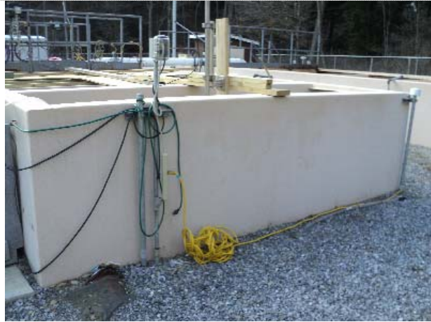
Photo 7: Nitrate Probe in Chlorine Contact Tank, Train B
