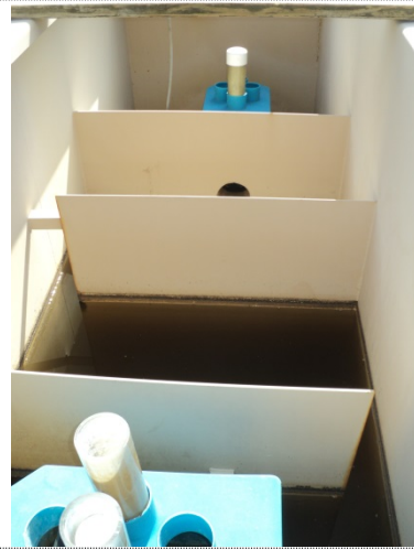
Photo 8: Erosion-type Chlorinator (near) & Sulfonator (far)
