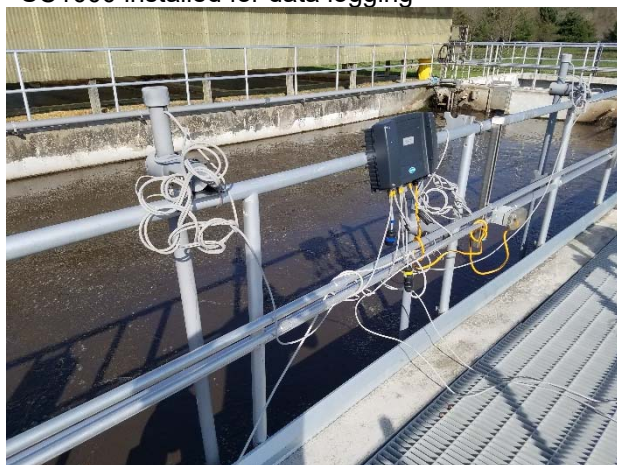
Second controller for aeration tanks
