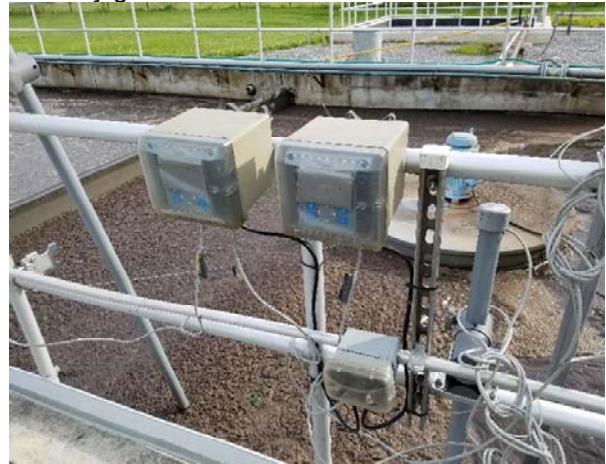
SC200 reconnected following on-site activities.
