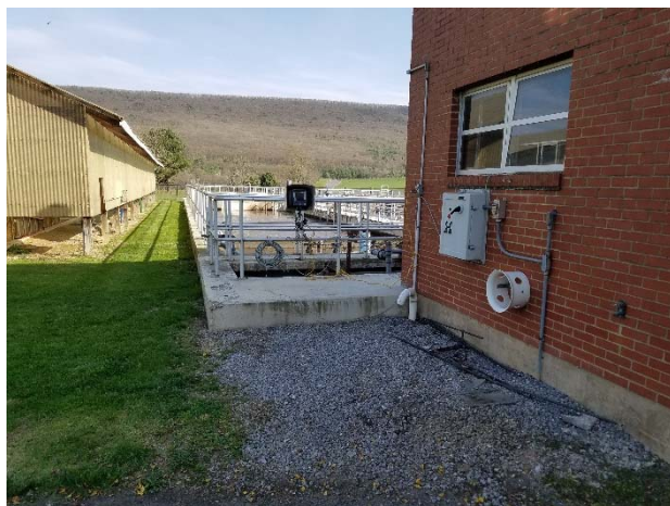
SC1000 installed for data logging
