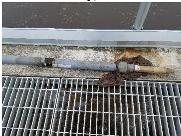
Photo 2: Immersion probe insufficiently maintained
