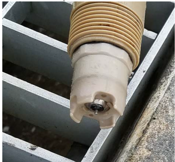
Probe tip, after cleaning, still has buildup on it.
