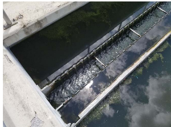
Photo 7: Algae in Secondary Clarifiers
