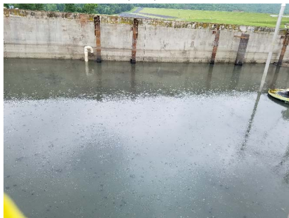
Photo 5: Off-gassing of waste in Equalization Tank
