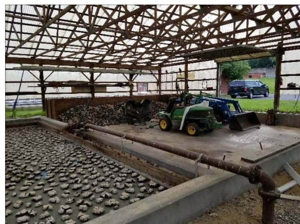
Photo 6: Solids Drying Facilities
