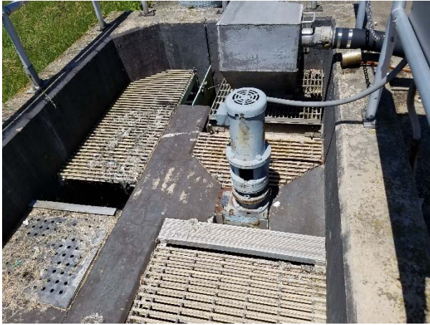
Old Comminutor at Headworks
