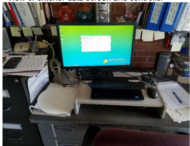
Data-logging monitor in control building
