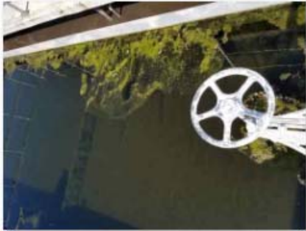
Algae growth in clarifier
