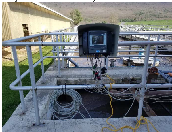
View of exterior data screen and controller
