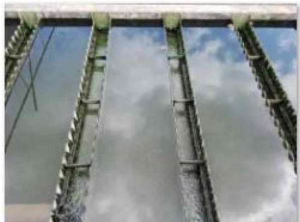
Secondary Clarifier Ashing
