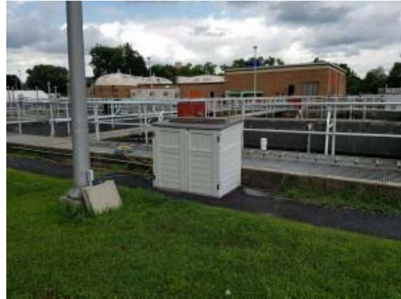
Mini-SCADA Housing for Aeration Probes
