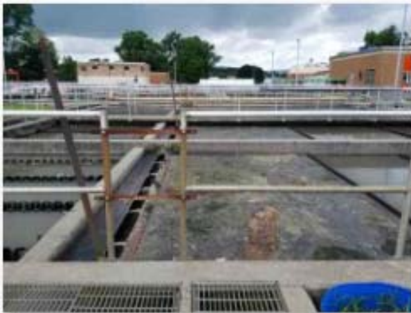
Primary Clarifiers & Scum Removal System
