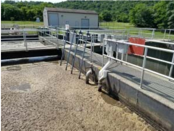
Aeration Tank Probes (DO, pH, ORP, TSS)
