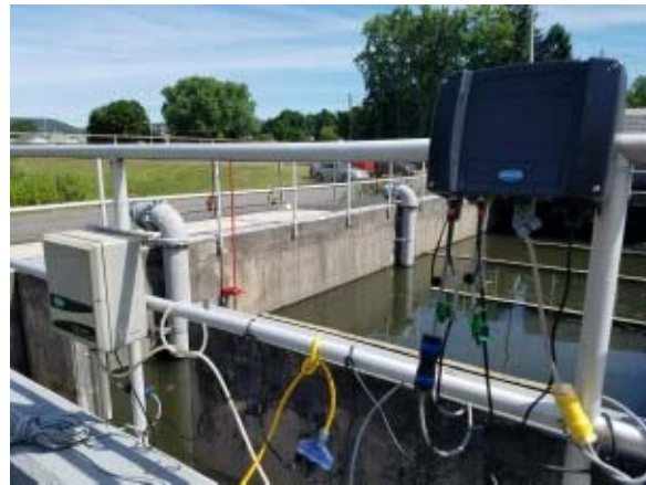
Effluent SC1000 & Cleaning System
