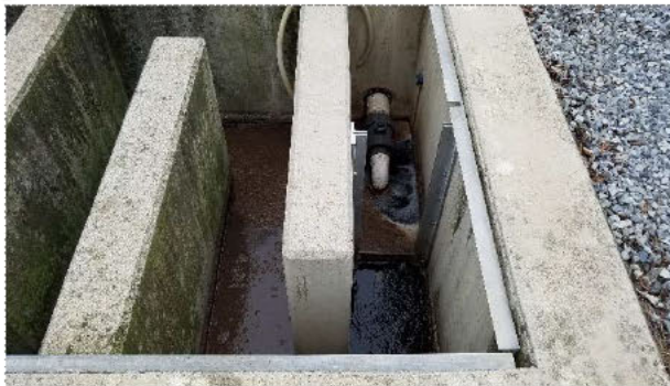
Chlorine Contact Tank, Influent End, solids present indicates carryover
