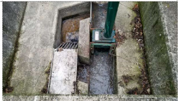
Headworks w/ Comminutor
