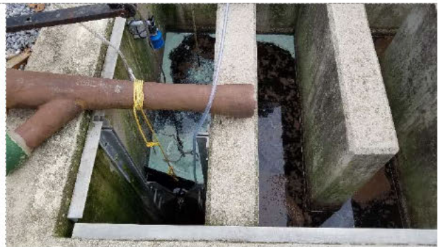
Chlorine Contact Tank, Effluent End—floating blue material are dissolved sulfite tablets
