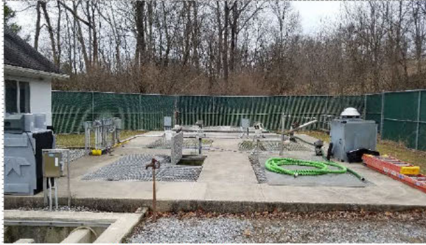
Overview of SBR Installation
