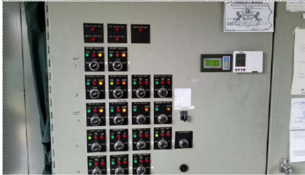
SBR Control: timer relays and switches
