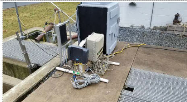
Effluent monitoring equipment
