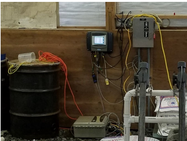
SC1000 Probe Controller & AISE Compressor
