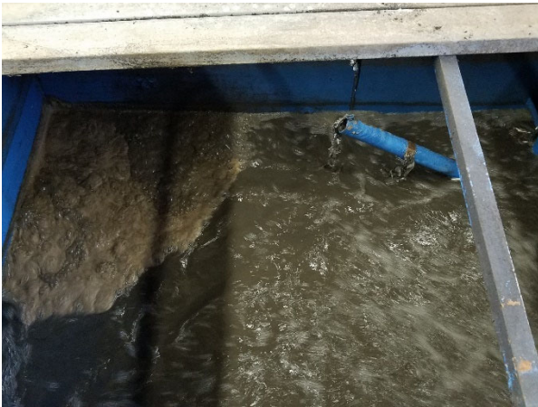
Sludge holding decant pipe
