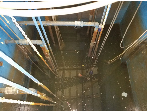
Effluent Wet Well
