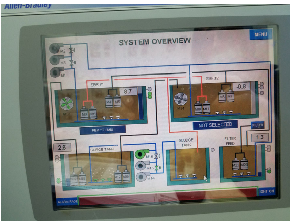
System overview on SCADA
