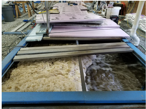
Sludge being wasted to holding tank.
