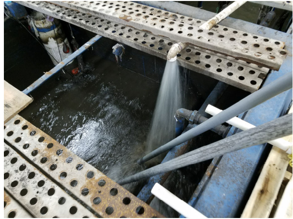
Influent entering SBR1 during fill cycle
