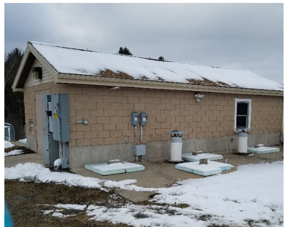
View of Amphidrome filter and building
