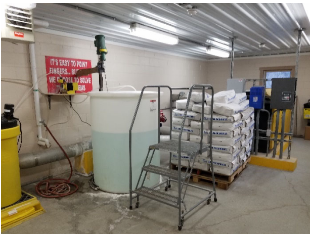
Sodium bicarbonate day tank & pump
