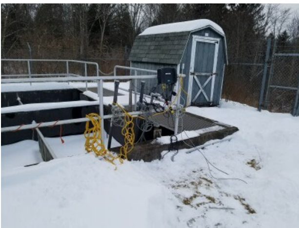
View of installed monitoring probes at effluent
