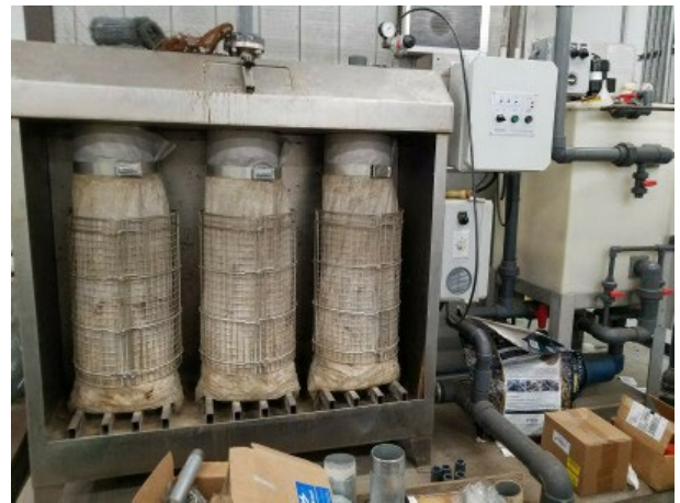
Biosolids bagging system
