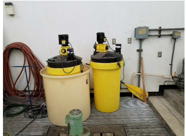
Chemical Day Tanks, unused
