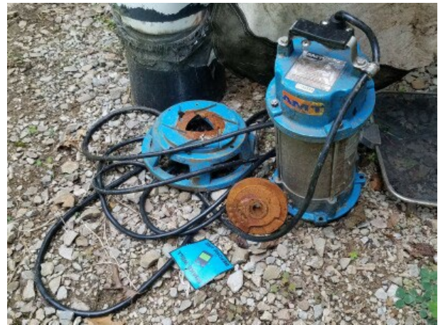
Rags destroyed this influent lift pump
