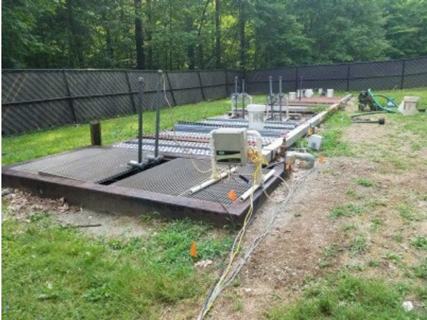
Treatment unit 1 and Surge Tank with probes
