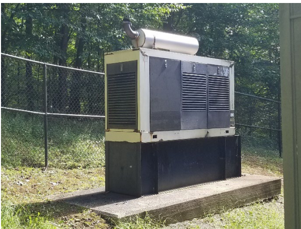
Generator needs another head gasket
