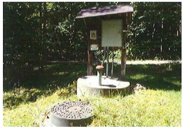
Pumping Station outside fence
