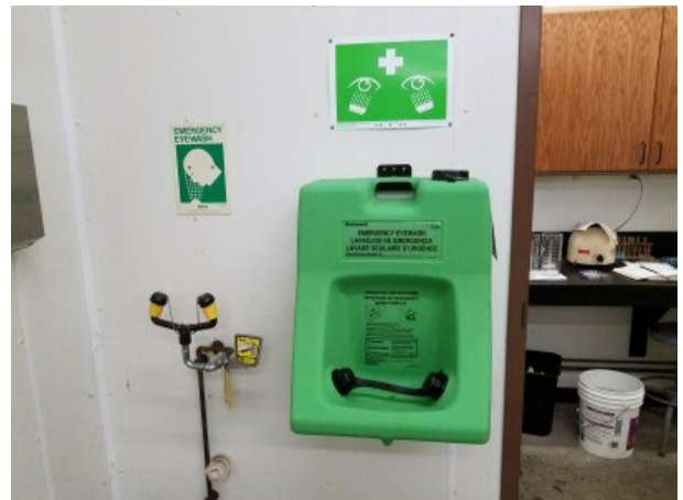
Temporary eye wash station next to nonfunctional eye wash station (due to water line break)
