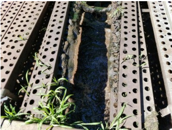
Solids accumulation on aeration tank
