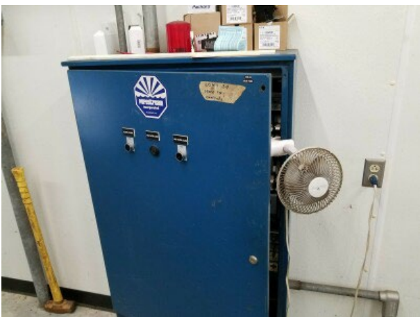
Secondary treatment plant control panel with temporary cooling fan
