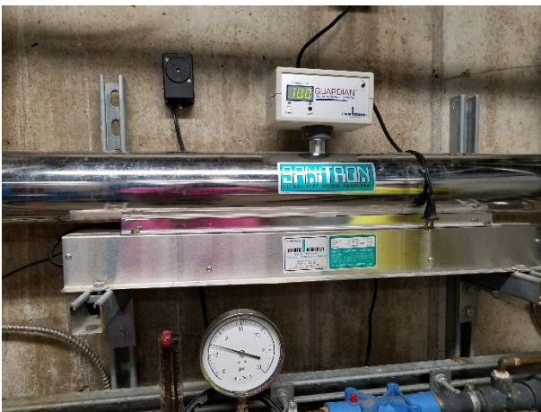
UV disinfection system
