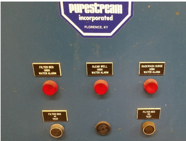
Filter control panel
