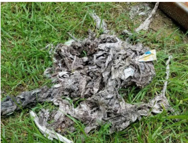
Material removed from pump impeller
