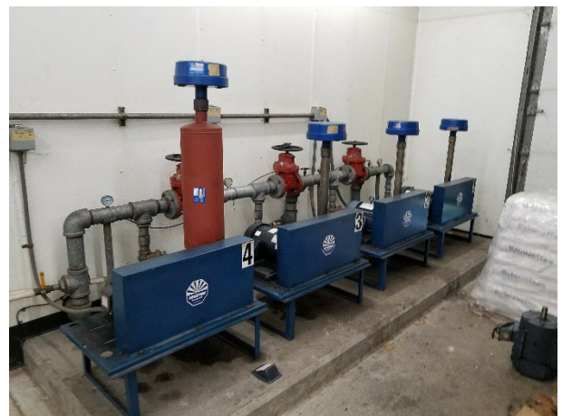
PD blowers for aeration and pumping
