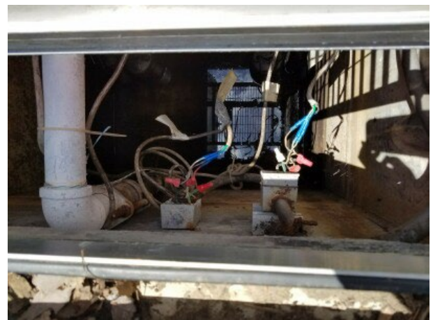
Unsecured electrical connections in wet well
