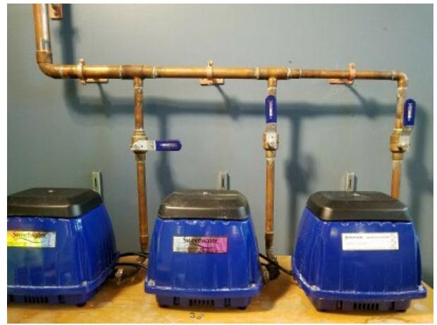
Air compressors for facility
