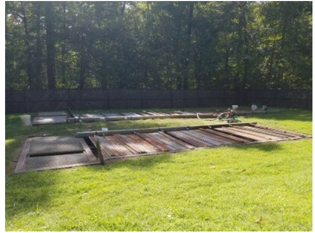
View of PureStream Secondary Treatment Plant
