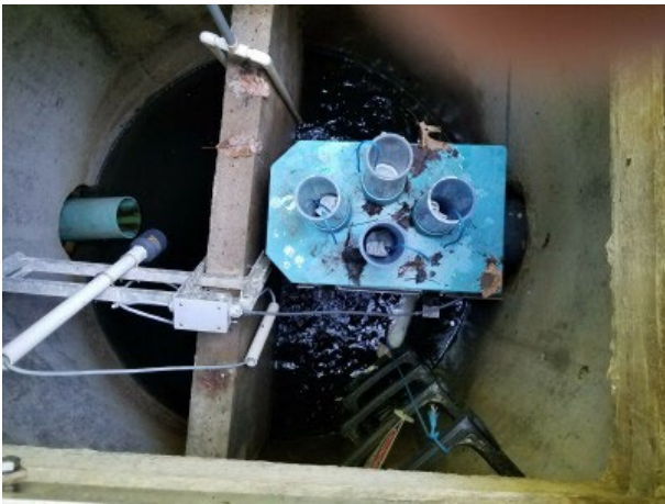
Sulfonator and Broken Ultrasonic Meter
