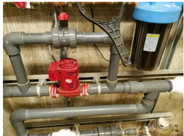
Pump and Filter
