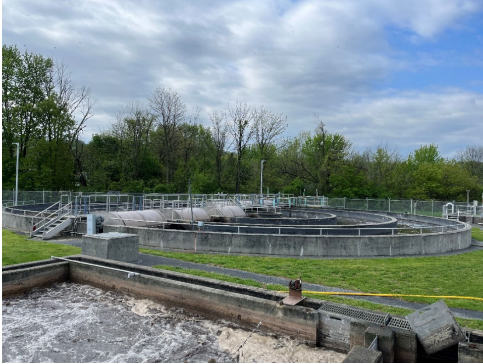
Overview of Orbal bioreactor, a 3-ring oxidation ditch arrangement aerated by brush rotors.
