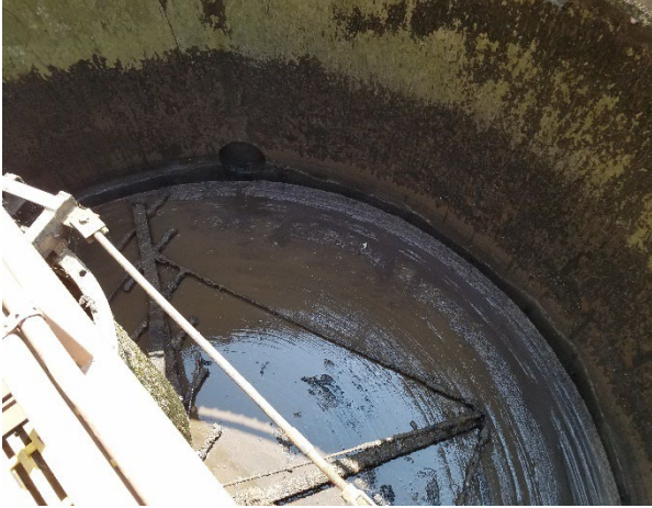
Clarifer Rake during down time
