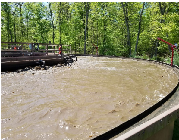
AER #1 high level due to small oriface between two aeration tanks
