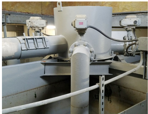
Filter #4 Distribution Box
