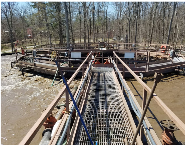
View across Aeration & Digester Tanks
