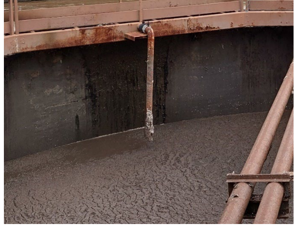
Broken air distribution line at digester
