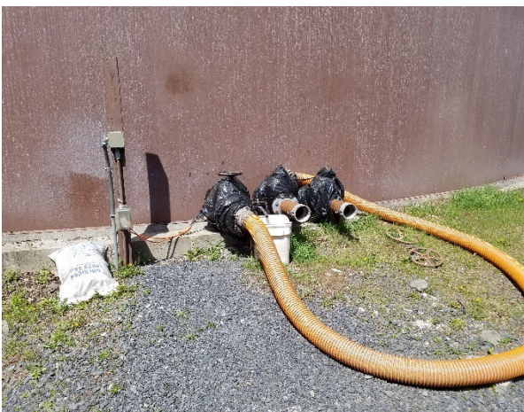
Tank Drain Valves at Grade
