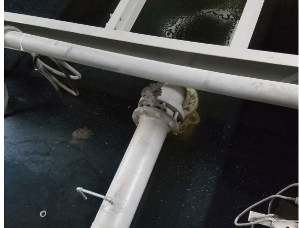
View into a filter unit
