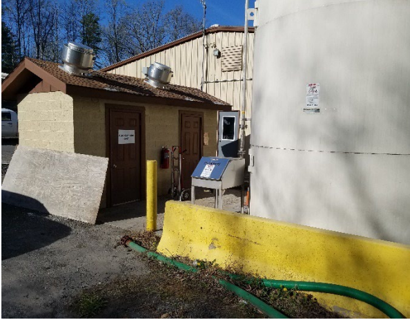
Methanol Tank, Effluent Sampler, Sulfonator
