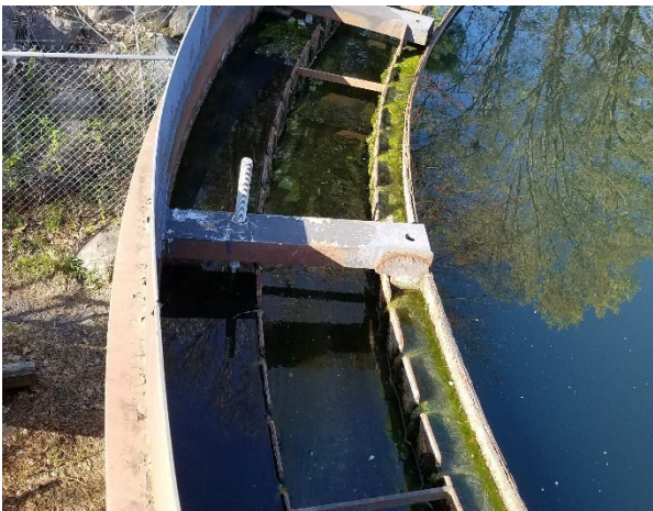
Algae in Clarifier Weirs
