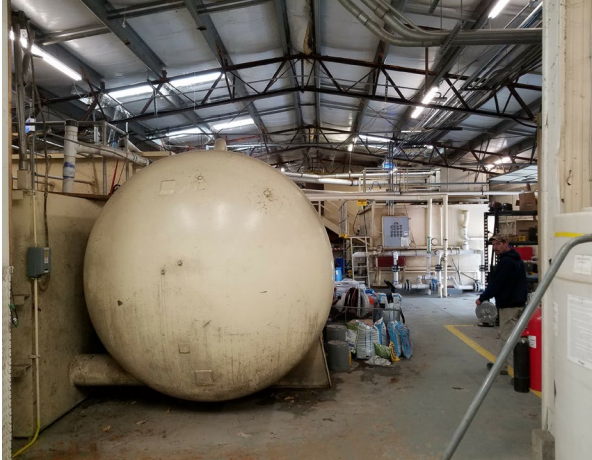
Inside Filter Building (Filters 1 – 3, Water Storage Tank)
