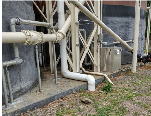
Rotary Lobe Blower installed to independently operate air-lift pumps
