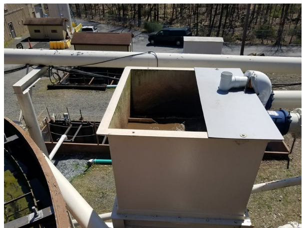
Sludge Distribution Box at Clarifiers
