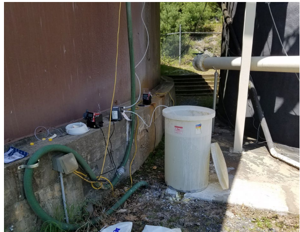
Temporary Soda Ash Day Tank
