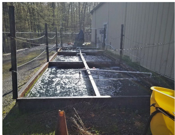
Hypochlorite Contact Tank
