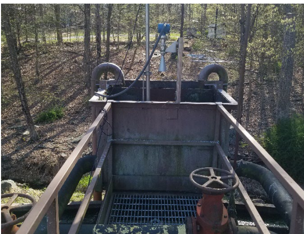
Influent Distribution Box w/ Flow Detection
