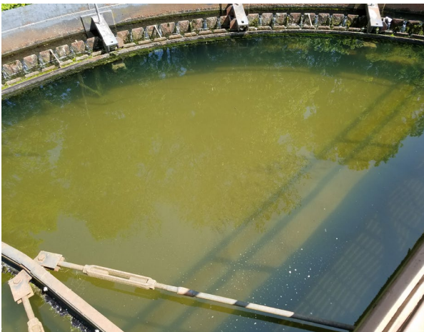
High Clarifier Blanket, pending increase in compressor size for air lift pumps
