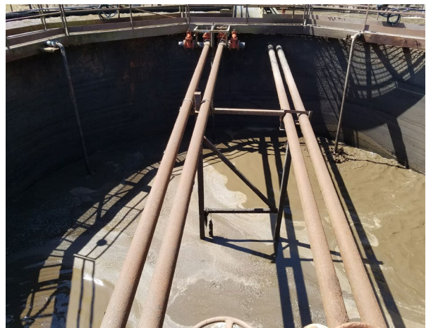
Sludge Holding / Aerobic Digester
