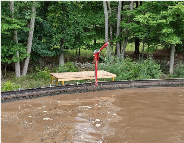
Jack Stand for Chopper Pump (1 of 4), with temporary platform for maintenance
