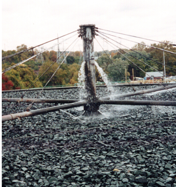
Figure 3.1 Tickling Filter with Leaking Seals
