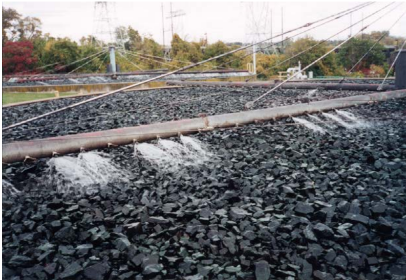
Figure 3.2 Tickling Filter with Clogged Nozzles
