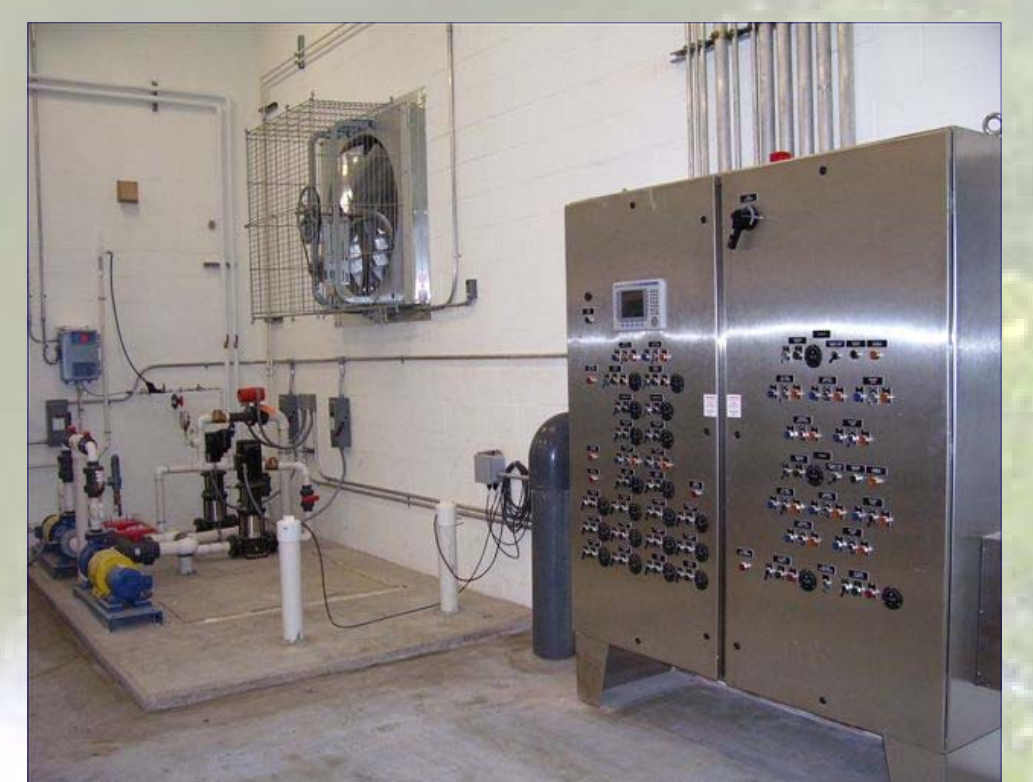
Backwash & Service Pumps; Control System
