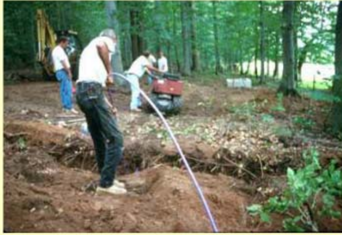
Drip tubing being installed with a vibratory plow in a wooded area
