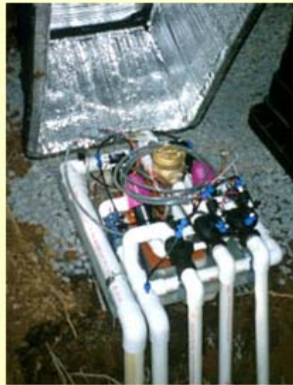
Hydraulic unit with conveyance lines
