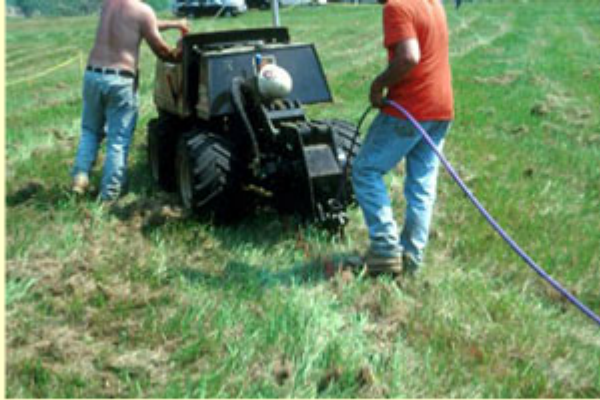
Drip tubing being installed in an open field using a vibratory plow
